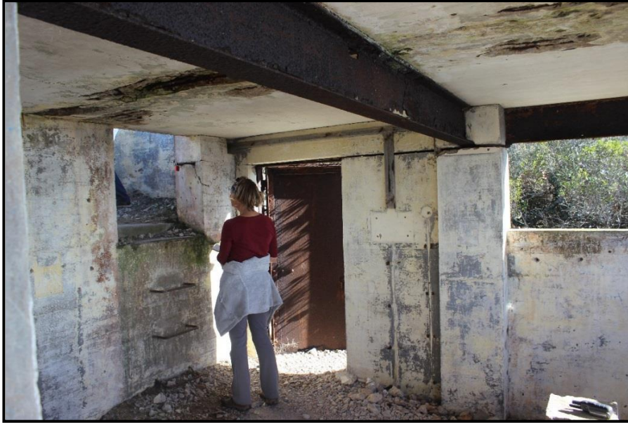
Figure 18. Site B. Interior showing the doorway, roof beams and stairway (ECU Photograph).
