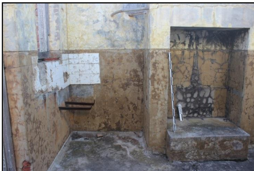
Figure 22. Site E kitchen with a fireplace and stove or sink below tiled façade (ECU Photograph).
