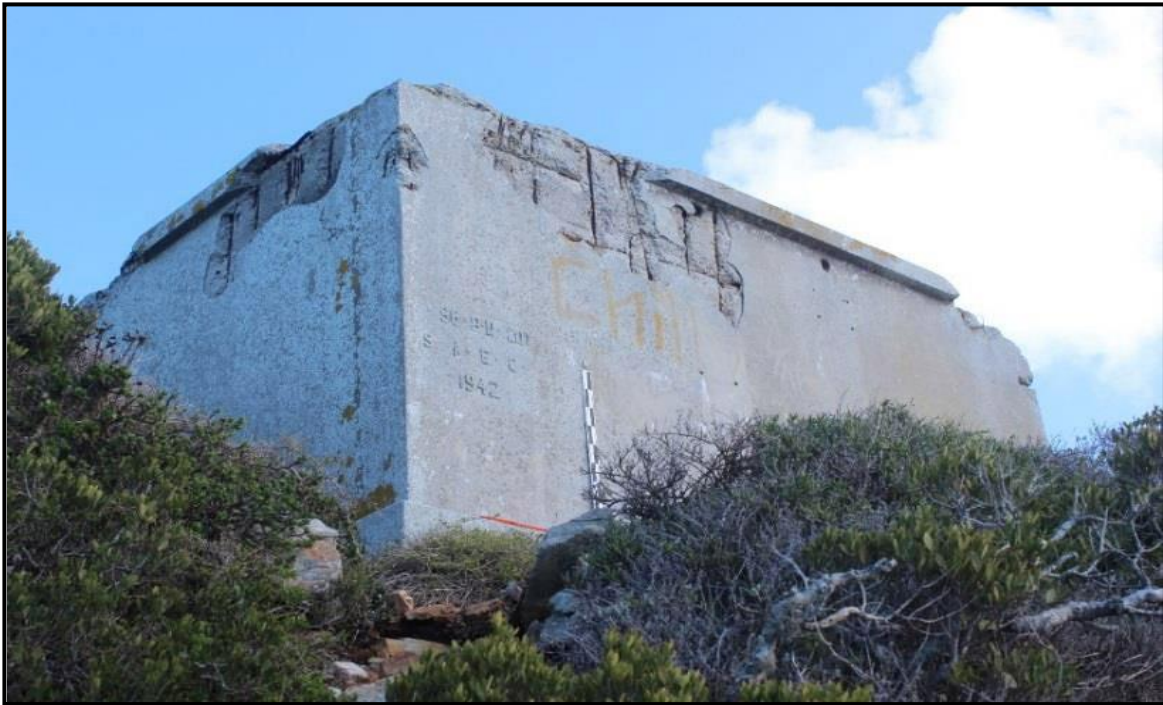
Figure 20. Site C square structure made from cement and rebar. Contains an inscription “S.A.E.C. 1942” (ECU Photograph).
